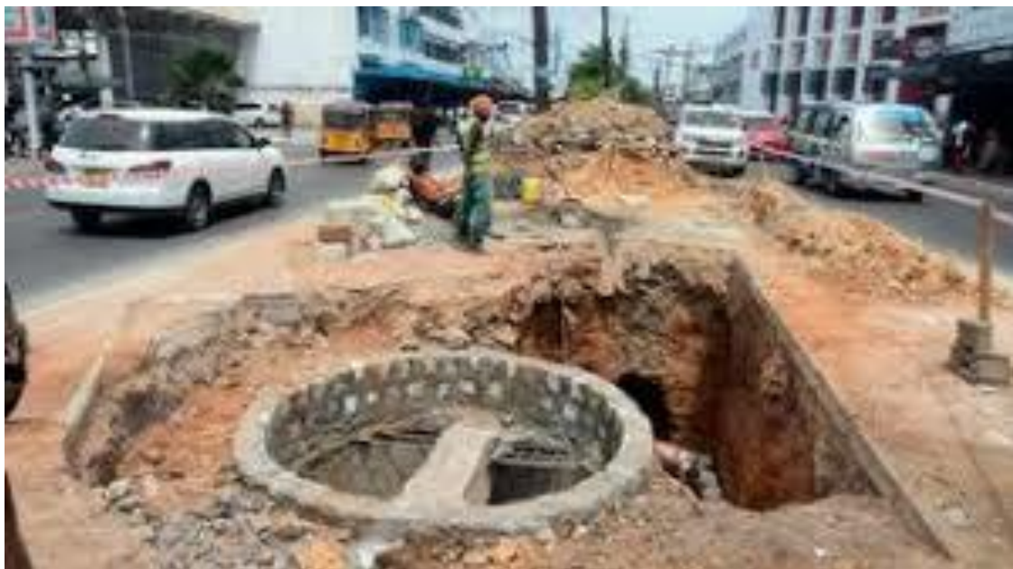
Danger posed by Mombasa's unfinished sewage projects
